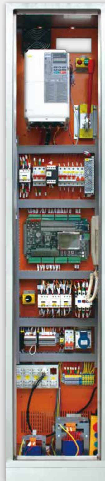
MRL CONTROL CABINET
