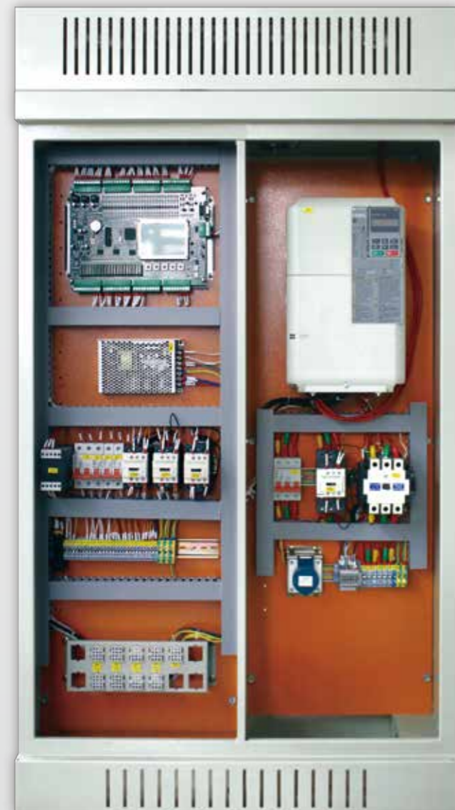
MR CONTROL CABINET
